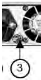
Figure 4-8. Unit Ground Connection
